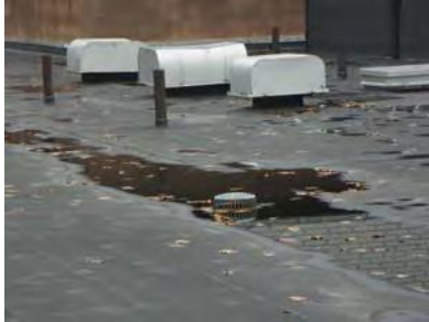
Ponding at roof drain
