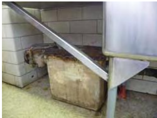
Grease traps to be replaced
