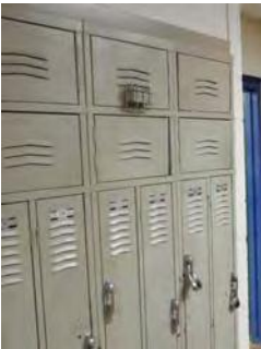
Pneumatic control located on upper locker
