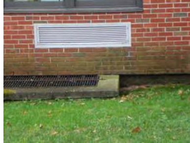
Mold on exterior wall
